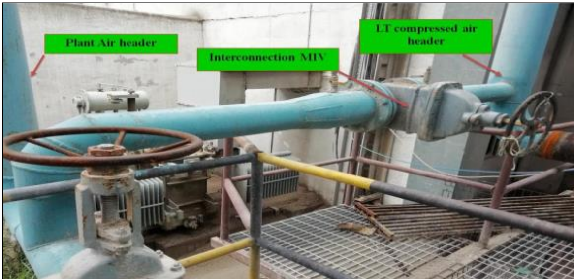
Figure 15: Compressed Air Optimization
