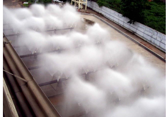
Figure 41: Mist Cooling Tower
