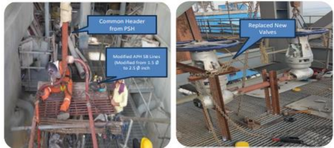
Figure 13: APH Soot Blowing
